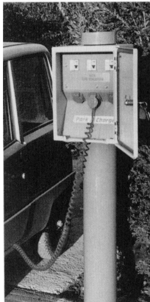
Fig. 8 : A three charging outlets column in Switzerland
