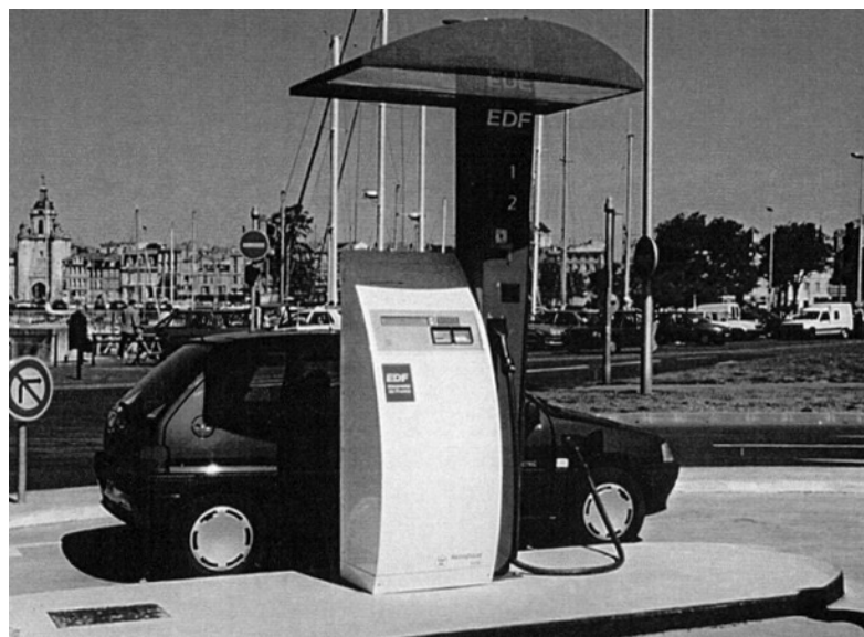
Fig. 4 : Fast charging station at La Rochelle
